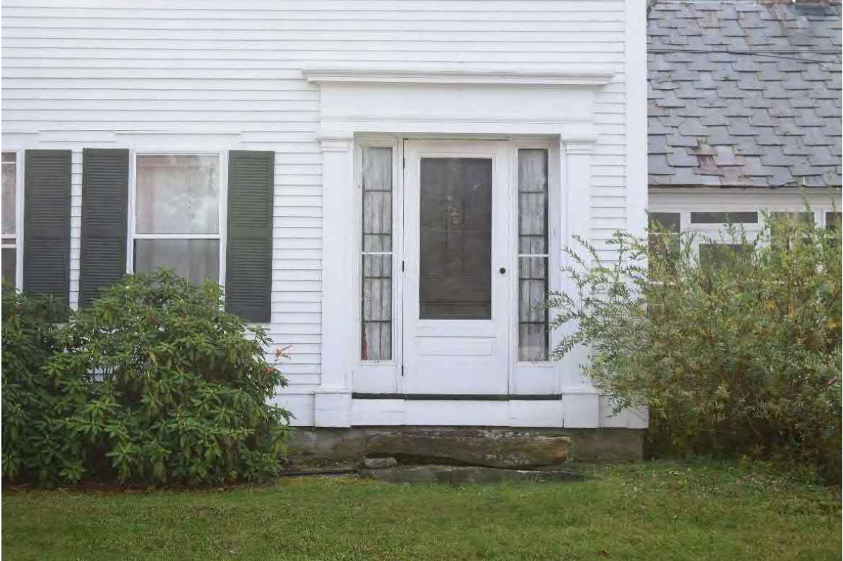
Photo 10. Granite steps at farmhouse associated with Structure 2 at 725 Main Street, facing southeast
